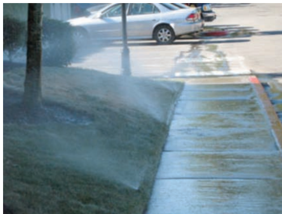
Slope in landscaping causing runoff
