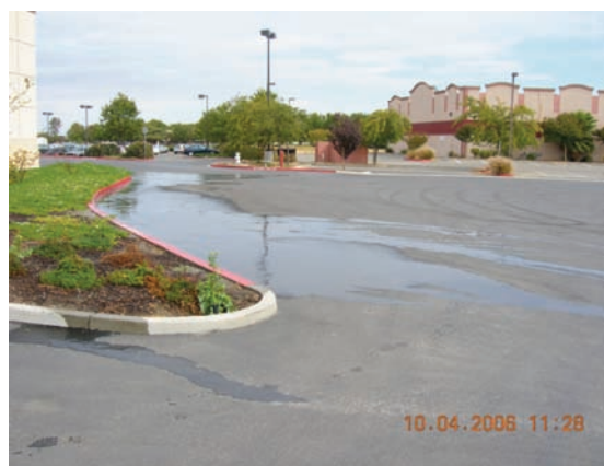
Standing puddle due to runoff
