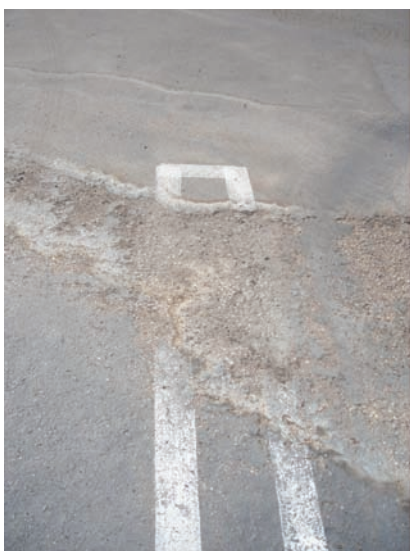
Damaged asphalt due to runoff
